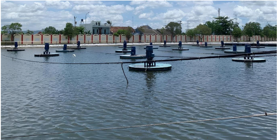
Figure 1. Main Pool Sewon WWTP
