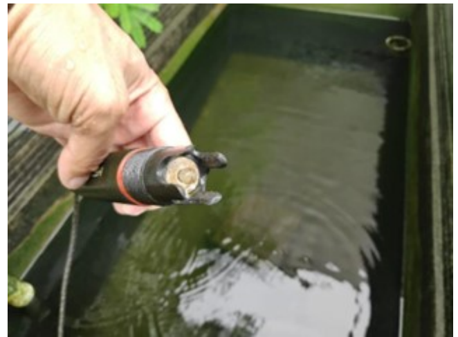
Figure 9 pH sensor condition after a few months of installation
