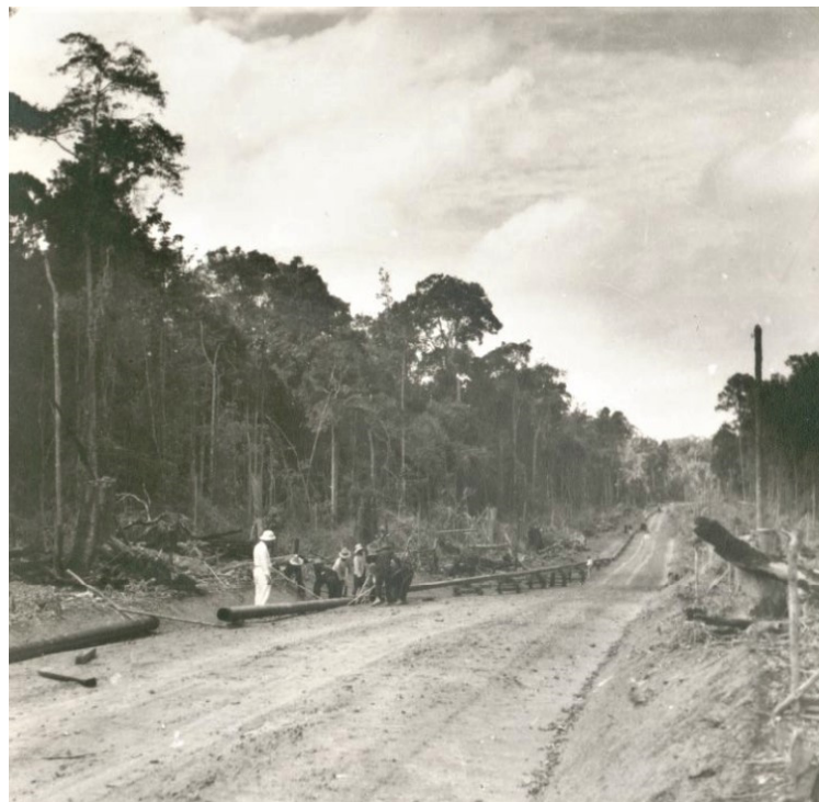
Figure 4. Construction of the Tempino oil pipeline with native workers, Jambi. Source: KITLV.
