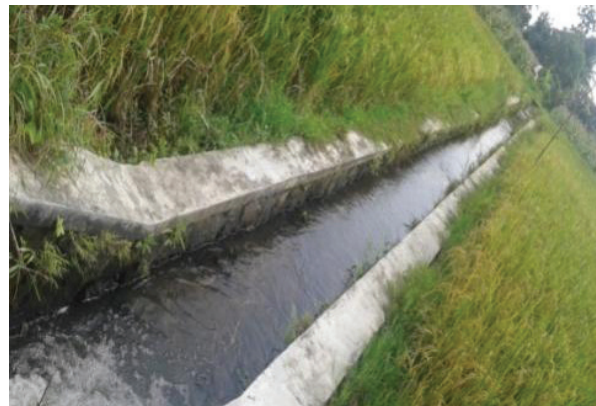
Figure 3. The Canal of Agriculture Irrigation Dam Kebo Kuning, has a function to deliver water irrigation from Dam Kebo Kuning to the farm field.
