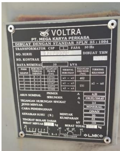
Gambar 2. Nameplate trafo SCG08-0066
