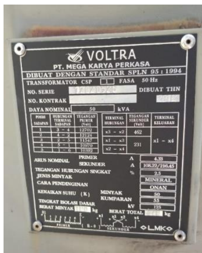
Gambar 2. Nameplate trafo SCG08-0066
