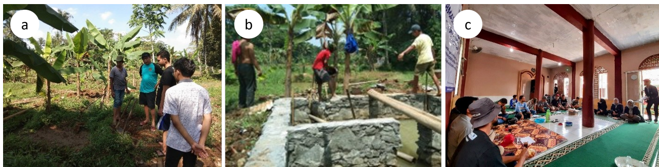
Figure 2 . (a) Initial construction site (beside irrigation canal); (b) Infrastructure development process; (c) Sharing knowledge about fish farming
