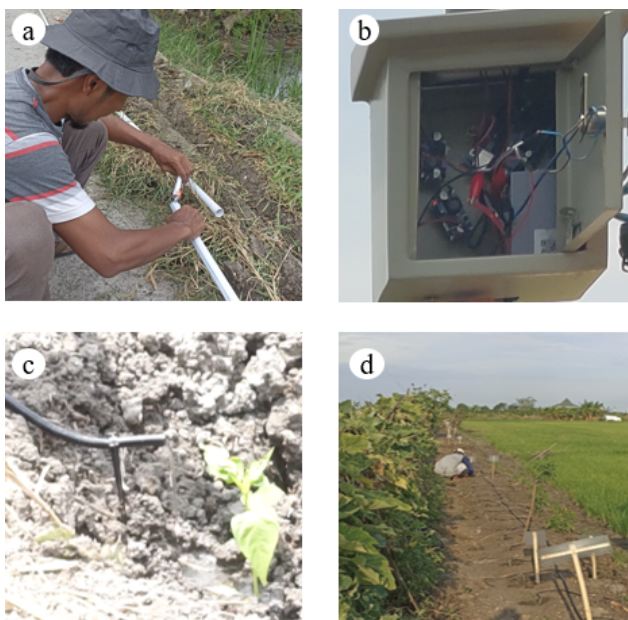
Figure 3. Installation of water installations with automation: (a) Installation of pipes for water flow from water sources to water reservoirs; (b) Installation of automation; (c) drip irrigation; (d) Installation of drip irrigation with irrigation automation in chili cultivation
