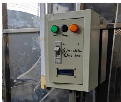
Figure 2. Bunker microcontroller control panel.
