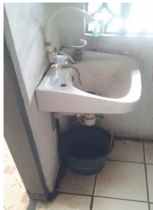
Figure 4.4 The location of the sink in the Water Resources Management Centre (WRMC) building
