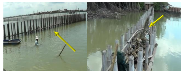
(a) Hybrid Low-crest Breakwater In Front of the Settlement and Mangrove Protection
