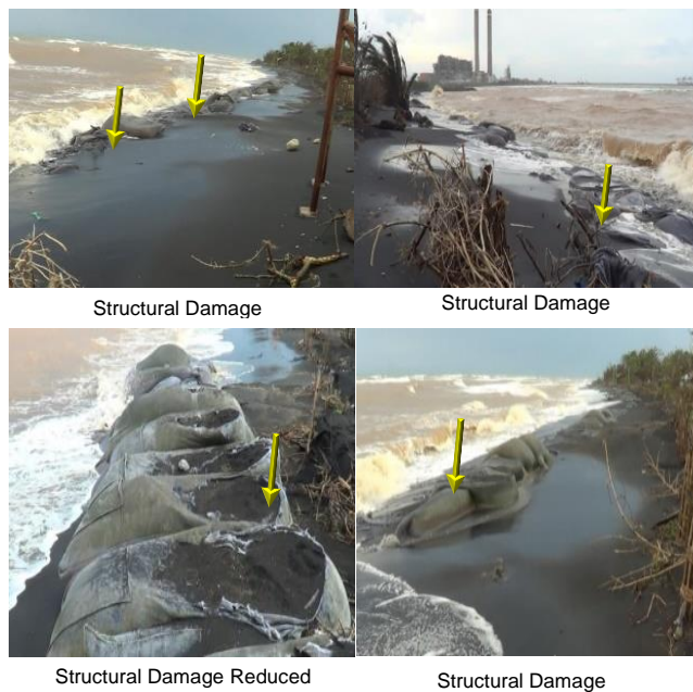
Figure 14. Structural damage of the low-crest breakwater structure on Jepara Regency
