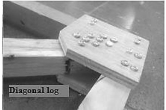
Figure 14. Failure on diagonal log of Truss 1 caused by tensile strength
