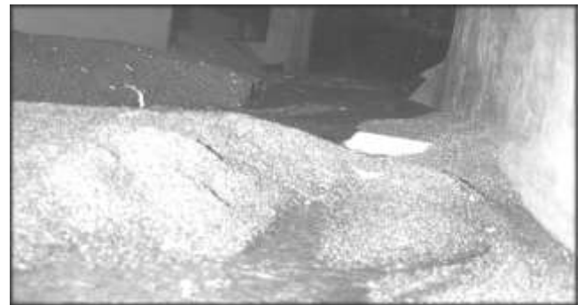
Figure 8. Material deposits due to sedimentation and erosion (non-scaled).
