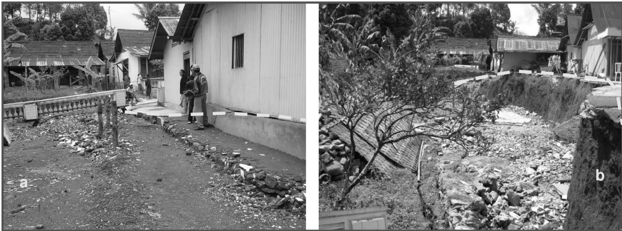
Figure 1: Crown of landslide (dash-line). (a) Cracks rose on 2 February 2009; (b) subsidence on 9 February 2009
