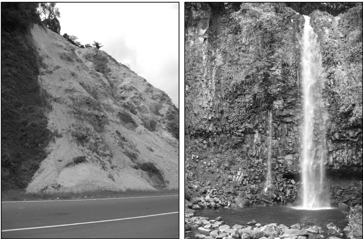
Figure 2: (a) Slope of weathered pumice tuff; (b) Fractured andesite in Anai Waterfall
