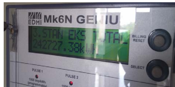
Fig. 9 The kWh meter that installed in SMG Sumba since July 2014.
