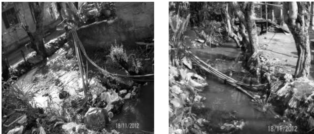
Figure 8. Water pipes crossing the stream
