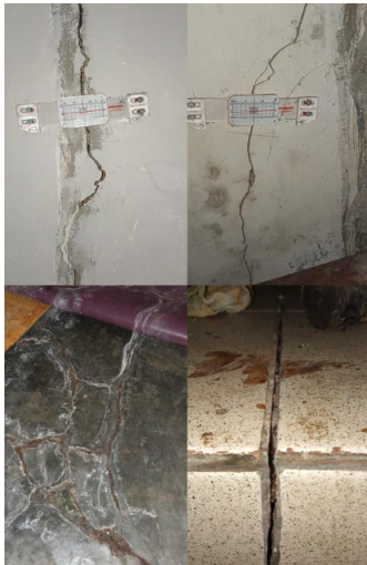
Figure 2: The effects of tunnel blast on residents' houses in Kompleks Tipar Silih Asih
